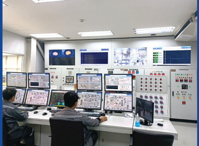
Incinerator system control room
