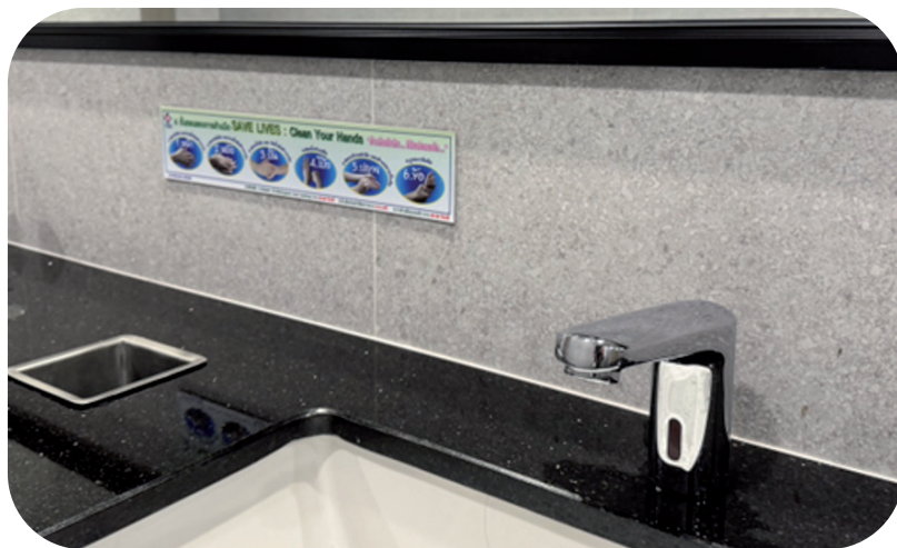
Installation of sensor-based water faucets and water conservation awareness materials within patient service areas
