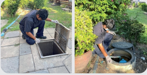
Regular inspection and maintenance of wastewater treatment systems to ensure effluent quality control
